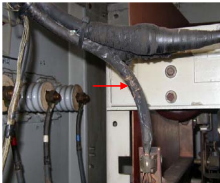
Figure-6: Severely deteriorated powder feed cable in 4160V switchgear cabinet displaying white powder and carbon tracks at arrow.
