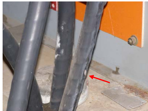
Figure-5: 13kV power feed cables showing corona powder and a small but intense area of tracking (shown at arrow).
