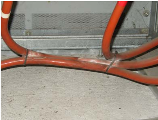
Figure-4: White powder/dust residue formed on 13kV power cables that are tie-wrapped together forming tight air spaces between each other; ideal locations for corona to form.
