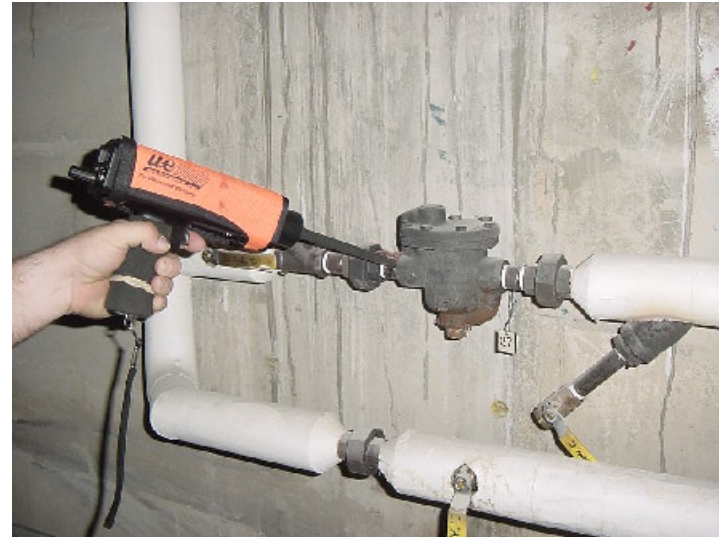
Ultrasound used to detect a trap leaking steam
