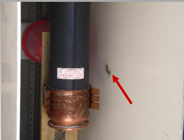
Carbon tracks on 13kV Load Interrupter Switch detected using ultrasound prevented catastrophic failure of component and lost production
